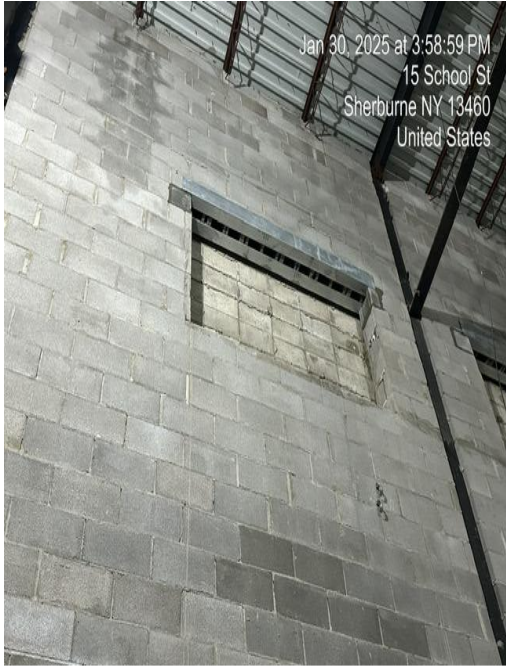
South Wall Ductwork Penetrations
